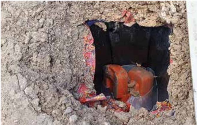
A broken well.
