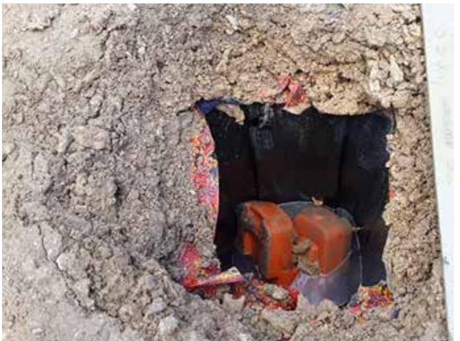
A broken well.
